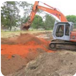
ViroSoil™ Technology can be used to remediate industrial sites. This site in Townsville was rendered safe and used for residential development.
