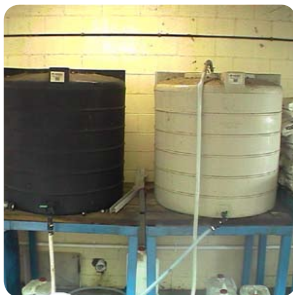
The pre-existing wastewater treatment plant at Beretta's Metal Finishing.
