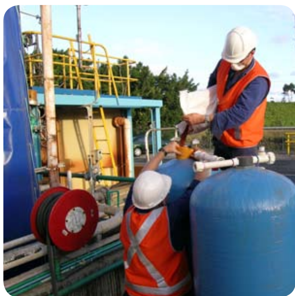
The reaction columns being manually packed by Virotec engineers and the fully commissioned ViroFilter™ Treatment System.
