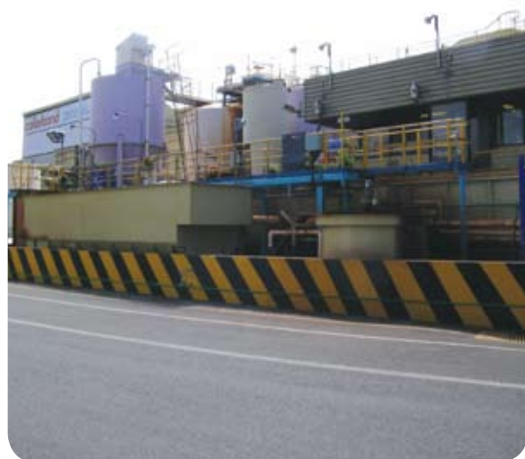
The existing wastewater treatment plant at the steel mill.
