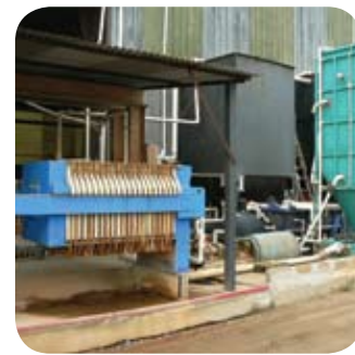
View of installed water treatment system
