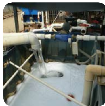
Treated water discharge.
