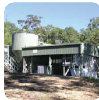
The wastewater treatment plant at the production facility of a large consumer goods manufacturer.
