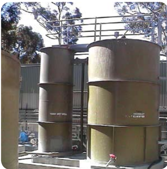
The secondary clarifier
