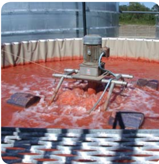
The ElectroBind™ mixing tank
