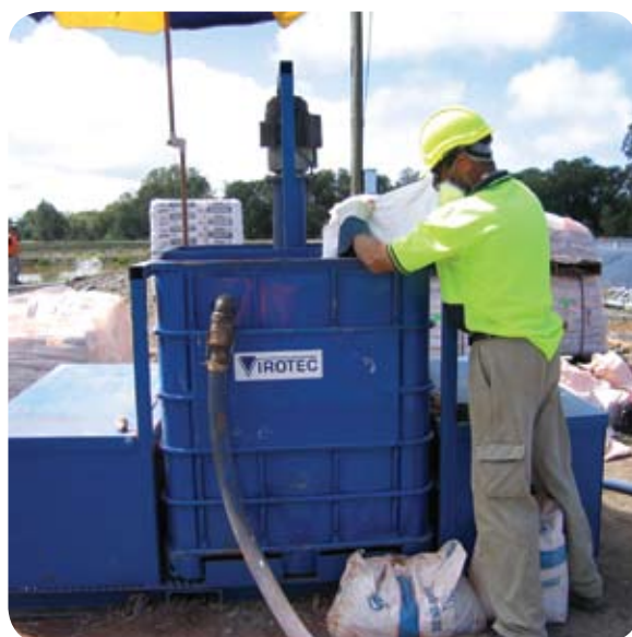
Treatment dosing plant used to mix the ElectroBind™ reagent in with the contaminated water so it can be sprayed back over the surface of the dam.
