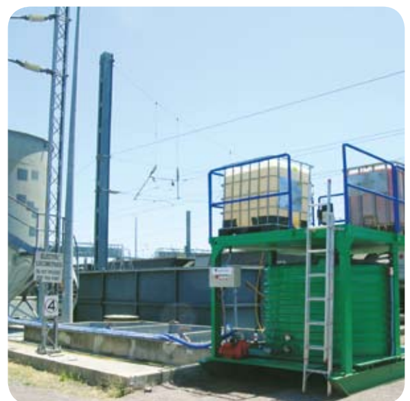
The ViroFlow™ Technology plant which treats waste water with ElectroBind™ reagent.
