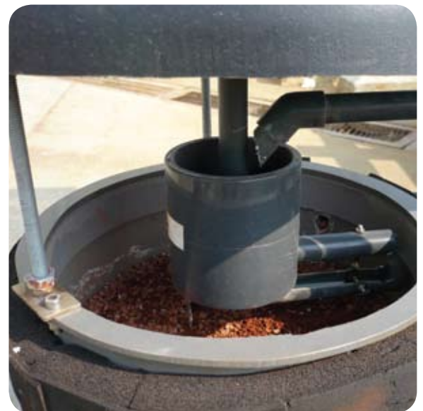
Close-up view of the ViroFlow™ Technology filter with acid- and iron-adjusted wastewater dispersed over the head of 2-6mm porous ElectroBind™ pellets.
