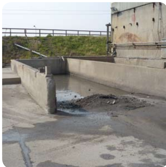
Two of the collection pits where the metal-contaminated site run-off is collected by mechanical sweepers prior to pumping to the holding lagoon.
