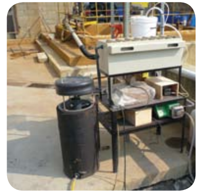
Contaminated site run-off was pumped from the holding lagoon to this ViroFlow™ Technology filter system, which included an iron and acid dosing phase, a solids' settling phase, and a filtration and metal-binding phase.
