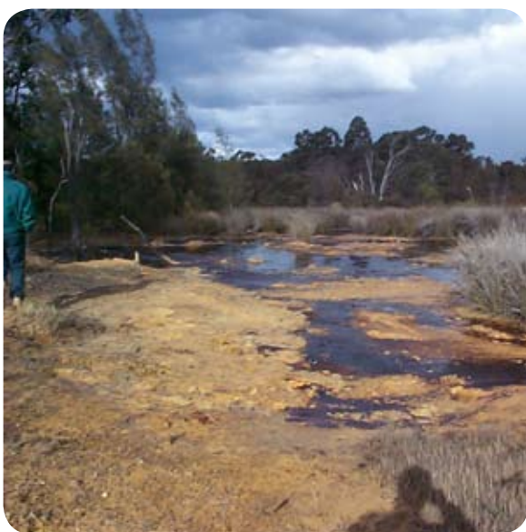
Dam seepage at Aberdare
