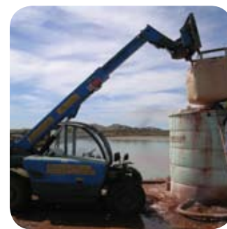
Addition of Acid B™ reagent into a mixing tank to produce a slurry that can be sprayed onto the tailings dam.
