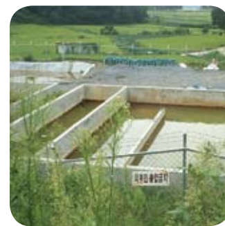
The ViroMine™ Technology filter system; Acid B™ pellets have been placed in the bottom of this filter (and another filter to the left) with a series of over-under baffles between the two filter beds.
