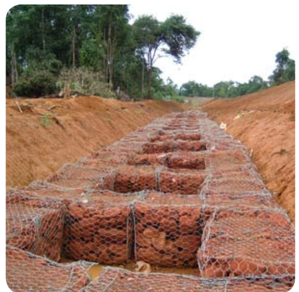
Permeable Reactive Barrier inside the Padan drainage gallery designed to treat contaminated runoff from the
