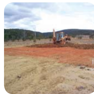
Terra B™ reagent being spread onto the zinc-enriched tailings with the backhoe.
