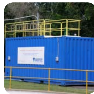
The ViroSewage™ Technology dosing plant at Fairfield Waste Water Treatment Plant.
