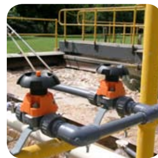
Dosing of ViroSewage™ Technology reagents at Fairfield Waste Water Treatment Plant.
