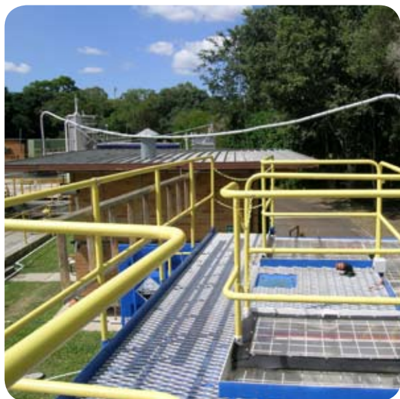
The ViroSewage™ Technology dosing plant adjacent to the Aerator Tank.
