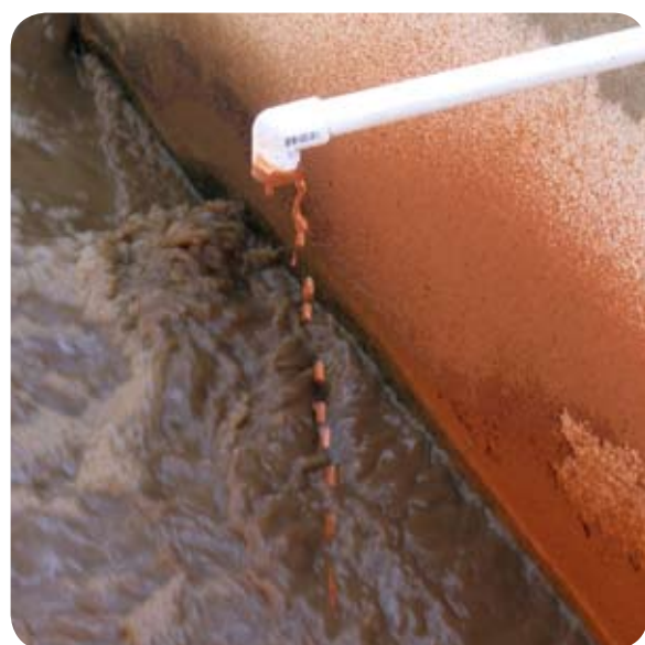
Dosing of ViroSewage™ reagents at Fairfield Waste Water Treatment Plant.
