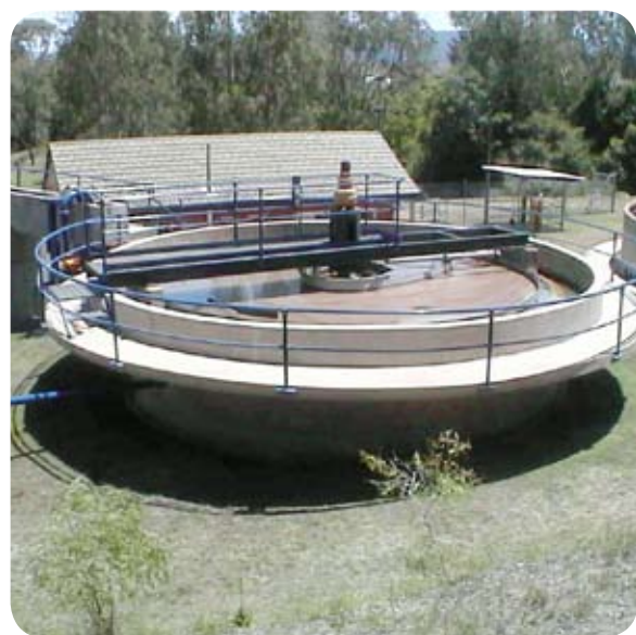
A component of the Kilcoy Sewage Treatment Plant.
