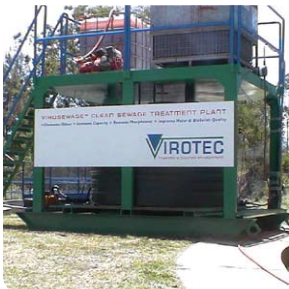
The ViroSewage™ Technology dosing plant at Kilcoy sewage treatment works.
