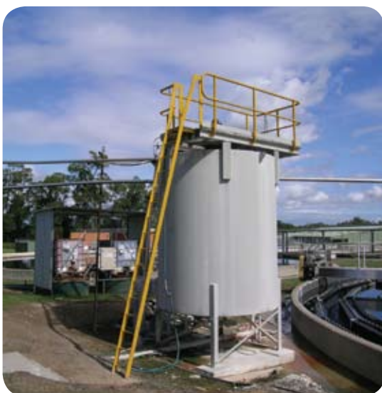
The Lime Clarifier
