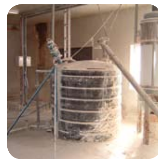
Lime batching plant at Redcliffe WWTP
