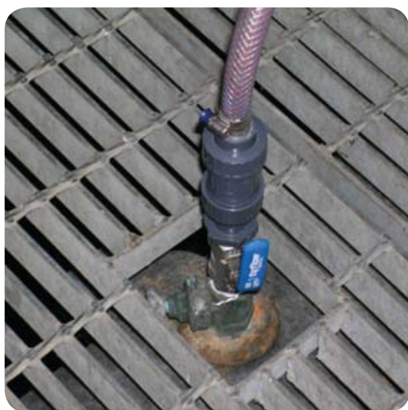
Dosing into sludge line
