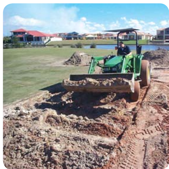
Top soil being applied to the area prior to turf being laid.
