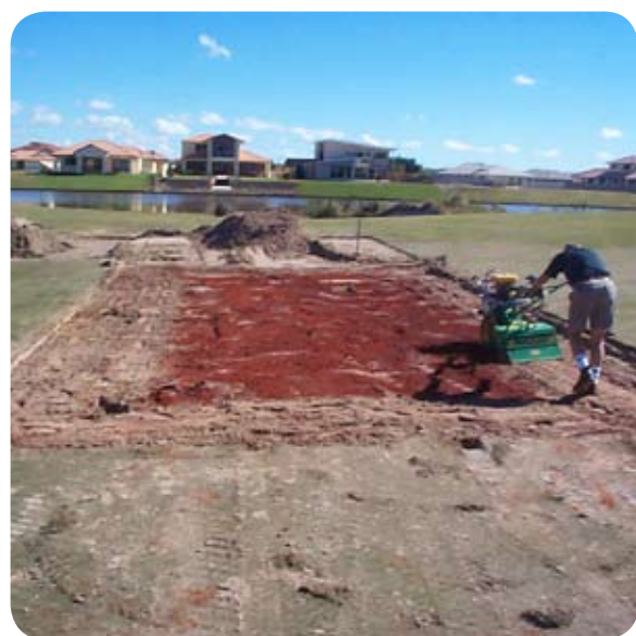
Mixing the ViroBind™ reagent into the sand and clay of the first treatment area by rotary hoe.
