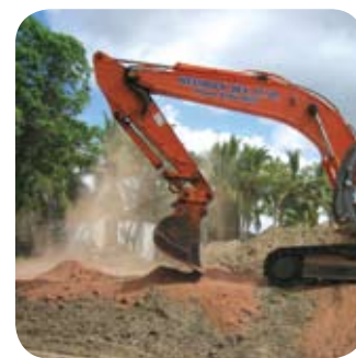
Mixing ViroBind™ reagent with contaminated soil at the Ross River site using an excavator.
