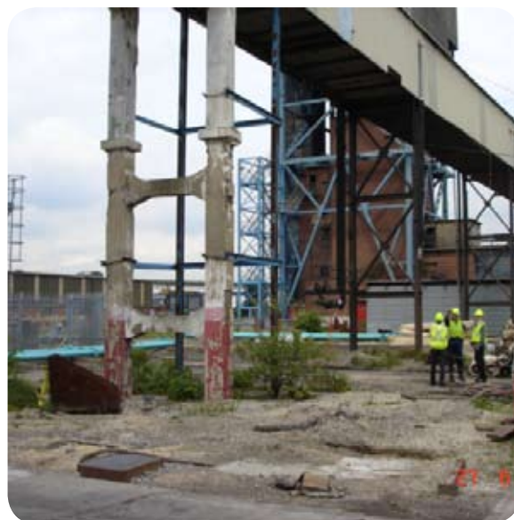
Site of ViroMine™ Technology treatment system at UK Coal’s Maltby Colliery site
