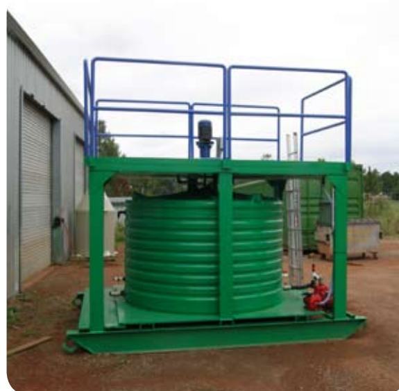
The Virotec Dosing Plant at Jilalan Rolling Stock Maintenance Depot
