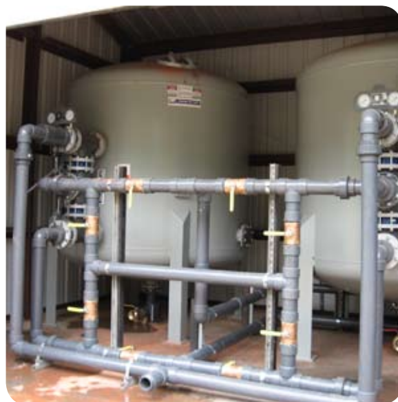
The filter installation at Gilbert-Summit
