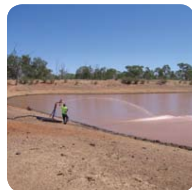
Dosing Acid B™ reagent as a 10% slurry into one of the five attenuation dams (note poor pre-treatment stormwater quality)
