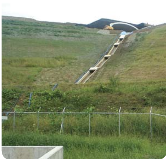
Stormwater runoff was channelled from the highway (top) via this drain (centre) to the ViroFlow™ Technology filter system (bottom) for treatment prior to discharge
