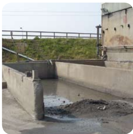
Holding bay where stormwater is collected before being pumped into the attenuation dam (behind rear wall)
