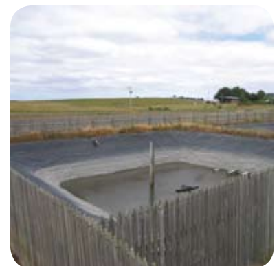
Stormwater drain, with strategically placed geotextile filter bags (right), treats runoff prior to holding in attenuation dam (centre)
