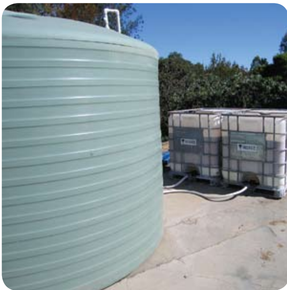
Stormwater holding tank (left) and two ViroFlow™ Technology filters (rear), with inlets at the bottom of the filters
