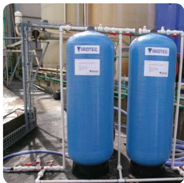
ViroFilter™ Technology can be designed to employ any upwardly or downwardly flowing filter configuration, of which this is an example
