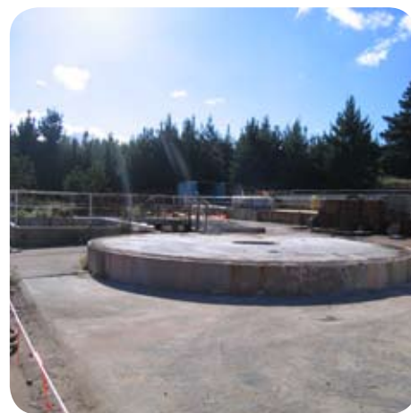
Typical underground storage tanks, often containing various types of liquid or solid waste, which require demolition and removal from site.
