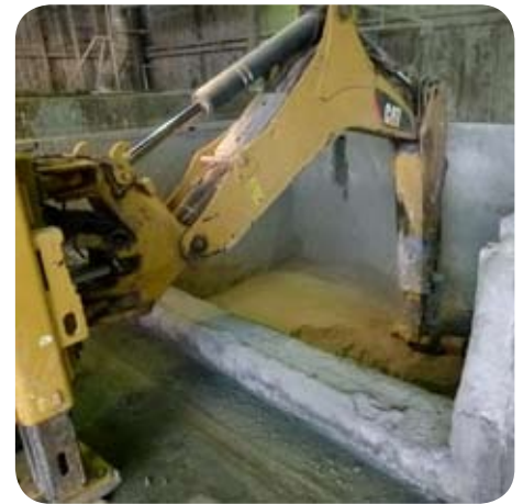
Contaminated demolition waste being treated with ElectroBind™ reagent at Virotec's Queensland facility.
