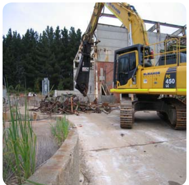
Cutting steel into smaller, manageable pieces suitable for safe transportation and processing.
