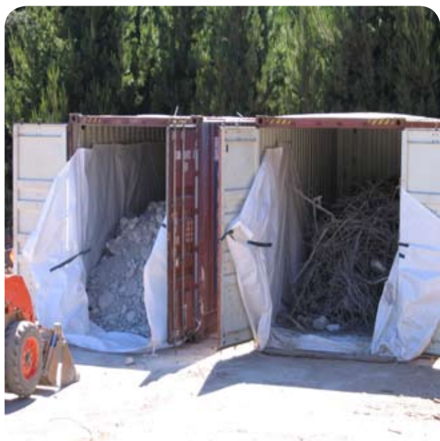
Crushed contaminated concrete and brick rubble (left) and chopped steel (right) loaded into lined shipping containers ready for removal and transportation to Virotec’s waste treatment facility.
