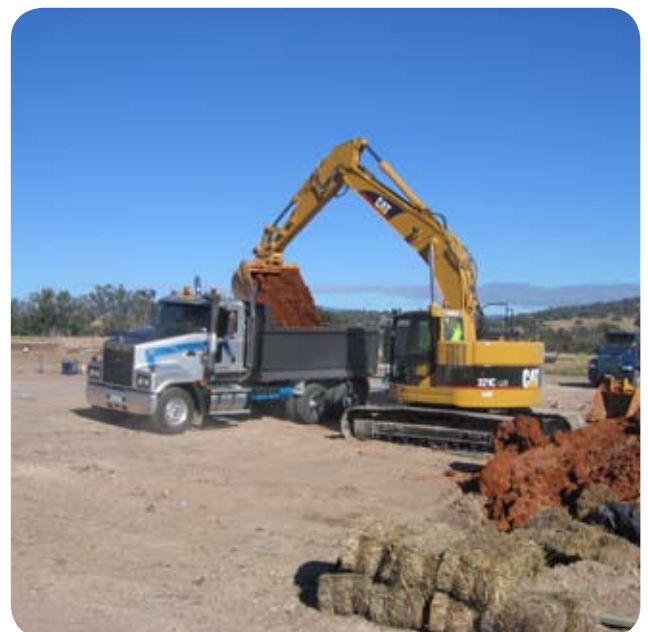
Treated demolition waste being loaded into semi tippers for transport to disposal site.
