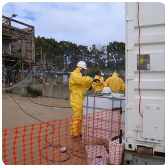
Virotec uses only state-of-the-art, industry-certified, personal protection equipment (PPE), such as that being used in this photo.
