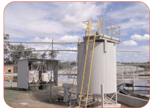
Figure 6: Dosing into lime clarifier (location 4)
