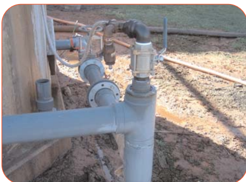
Figure 7: Dosing point (location 5)
