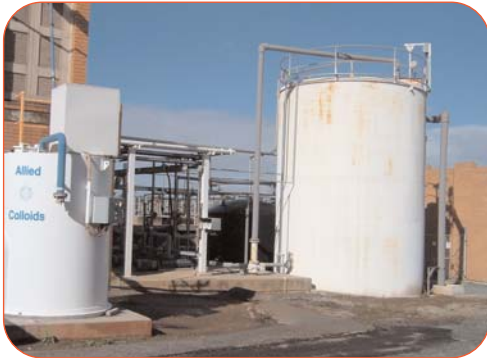
Figure 3: Day Holding Tank
