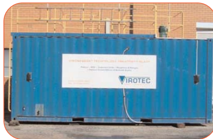
Figure 9: ViroSewage™ Technology dosing plant
