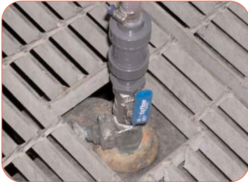
Figure 5: Dosing into sludge line (location 1)
