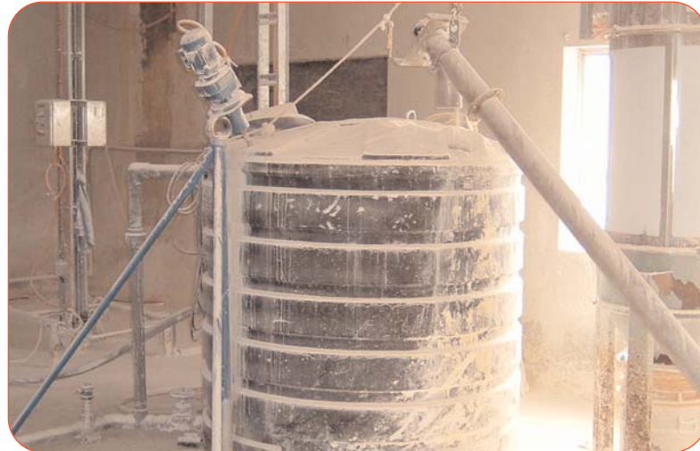
Figure 1: Lime batching plant at Redcliffe WWTP.
