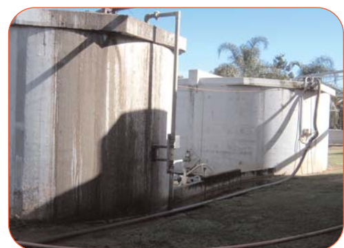
Figure 8: Final dosing into aeration tank
