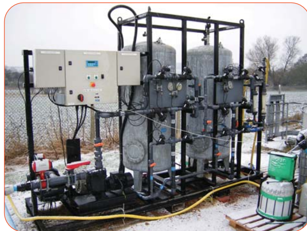
Figure 4: ViroFilter™ Technology Filter Pairing A
